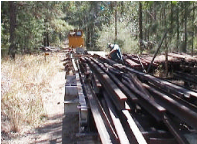
Left: Greg checking the newly stacked rails for transporting to the station area.
