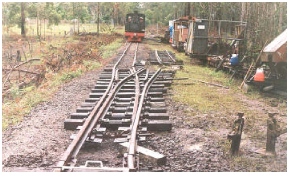
Points in position at the start of a wet day's work. The curve in the points was removed by jacking and barring across during the day. The panel of
