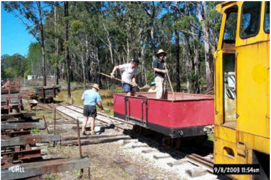
Ballasting the second set of points (No. 10) on 9 th September 2003. Herb Coleman and Greg Stephenson levelling ballast whilst Brian Wilson and Terry Olsson unload wagon. (Photo Ken McHugh)
