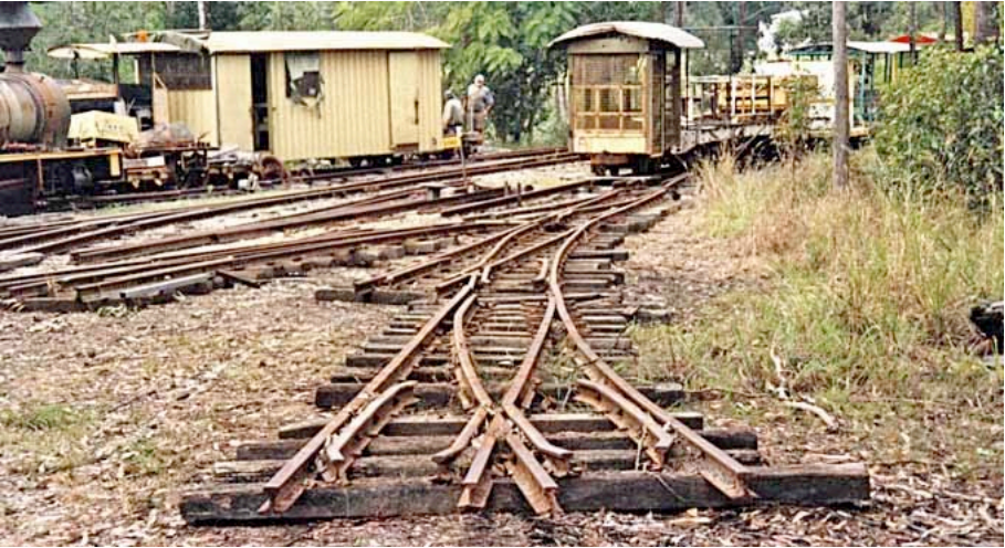
Pointwork roughly placed for the southern end of the passing loop and access to the compound. Bill Blannin photo [bb280_2]
