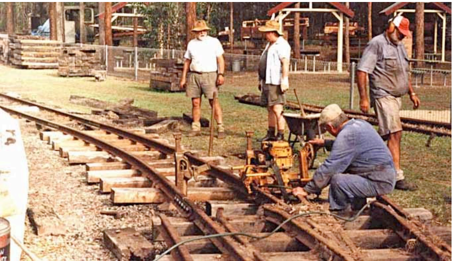
Points at Margaret Street end of passing loop - Leslie Beahan using motorised rail drill to drill fishplate holes to allow points to be connected to existing mainline. Bill Blannin photo [bb280_1]
