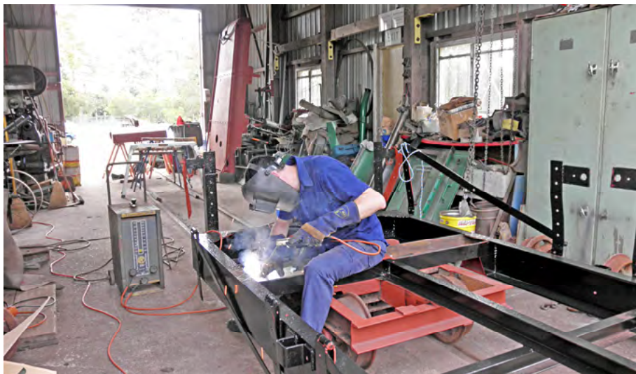
Mark Gough replacing rusted sections on the Nambour work wagon. Bob Gough photographer.
