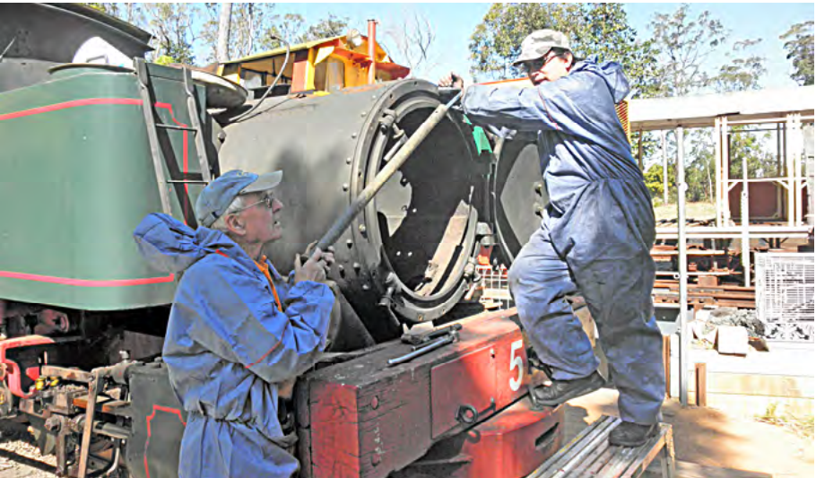
Bob Gough & Brad Bell removing rusty nuts & bolts from smoke box door ring on Bundy No 5. The ring & door were later removed to storage. Mark Gough photographer.
