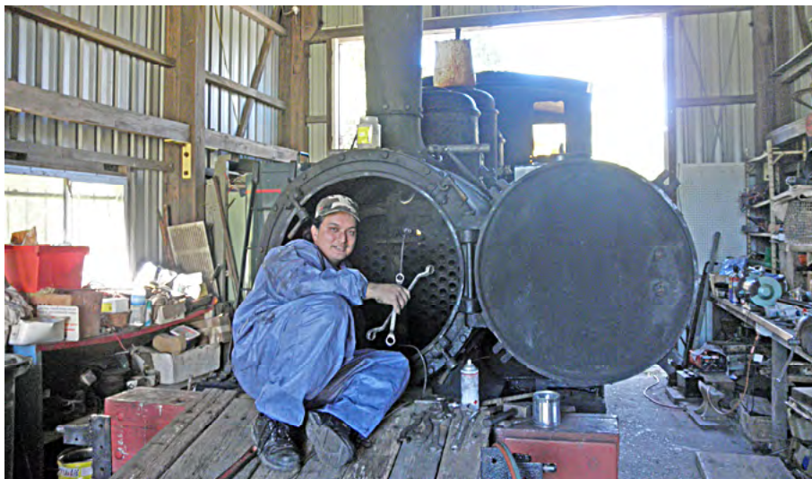
New member Brad Bell works on Bundy No 5, helping to dismantle the loco for new tubes and other work, 30 June 2012. Bob Gough photographer.
