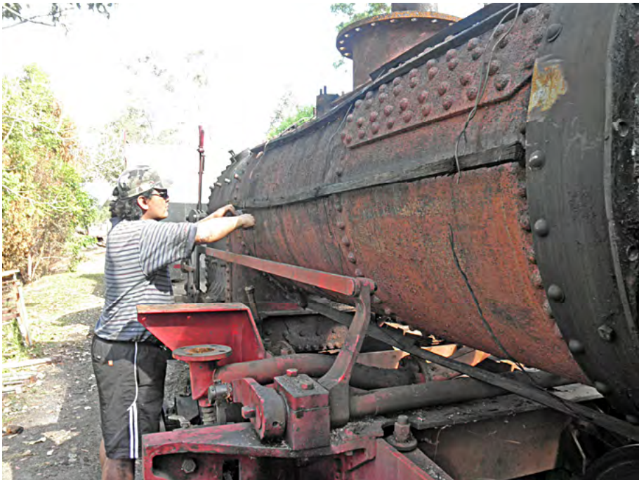
Brad Bell removing cladding support timbers from Bundy's boiler during the work party, 29 September 2012. Bob Gough photographer.
