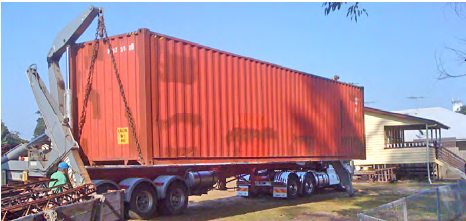
The Mens Shed storage container being unloaded into its temporary location near the picnic area, 17 December. Geoff Westcott photographer. [gw_013]
