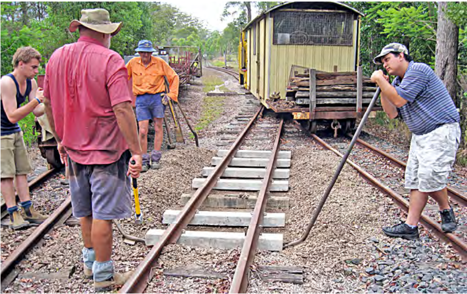
Installing Mackay concrete sleepers in crossover to Workshop, 5 January 2013. Terry Olsson photographer.
