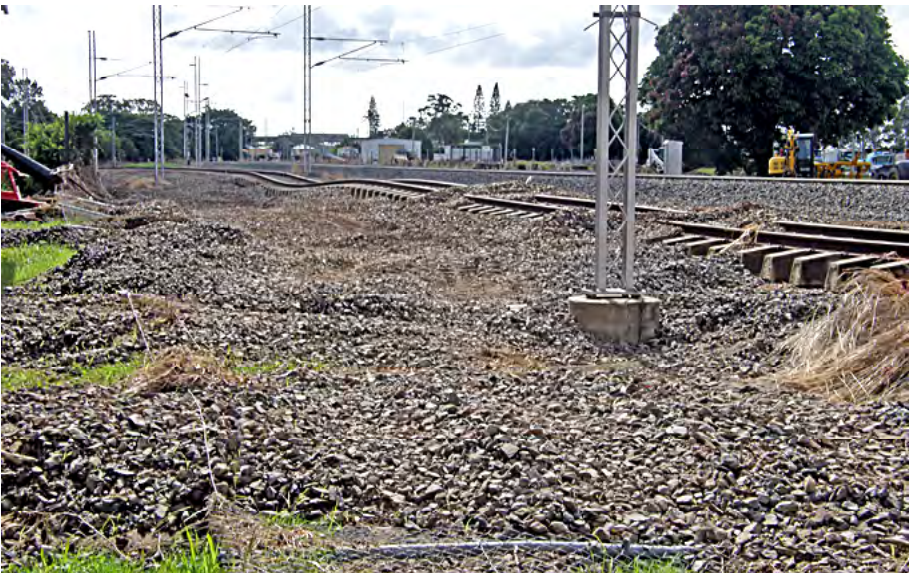
Part of the many tons of ballast washed from the North Coast Line into the Bundaberg Railway Museum precinct. Graham Hibberd photographer.
