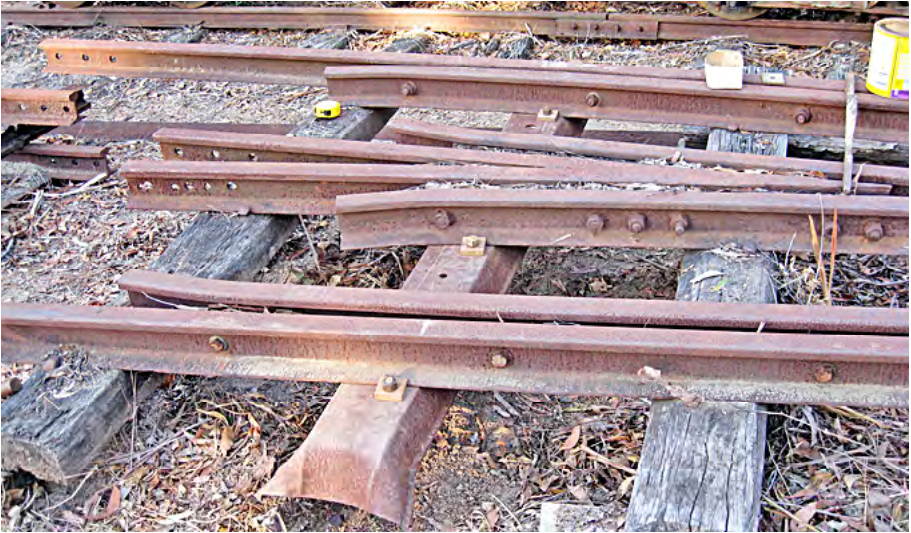
First steel sleeper in points for New Storey Brook crossing loop. Terry Olsson photographer.
