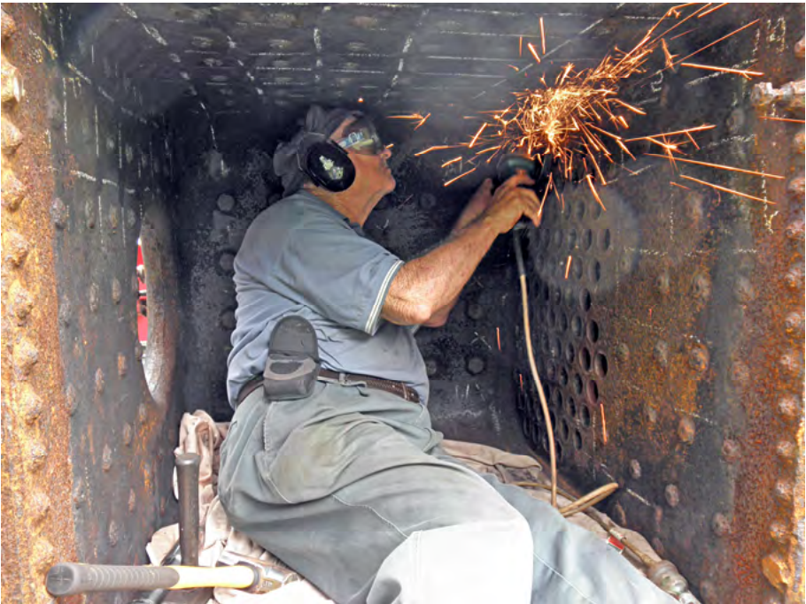
Bob Gough in the fire box of Bundy No 5, grinding the ends of the boiler tubes so that they can be removed. Mark Gough photographer.
