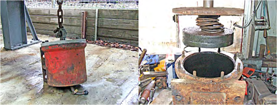
One of the brake cylinders sitting on the pit floor (left). Without the pit this job would have been more difficult and taken longer. Cylinder top removed (right) to reveal built up dirt oil and a well used spring. Mark Gough photographer.
