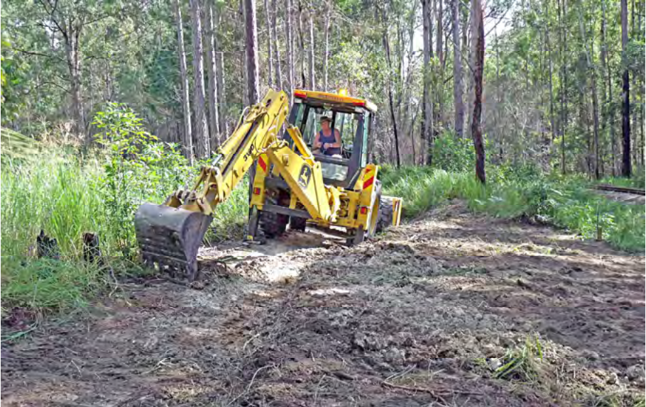
Ralph Cumner digs the open drain which will divert stormwater away from the mainline construction area at Storybrook Station, May 2013. See report inside. Greg Stephenson photographer.
