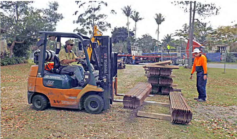
Tony Lindsay operating the CRT Woodford Country Store's forklift to complete unloading of steel sleepers. Due to limited off-road capability of the forklift, they were placed into a temporary stockpile. Greg Stephenson photographer.
