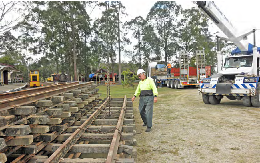
Unloading some of the fifteen panels of rail on concrete sleepers transported from Ingham, 26 August 2013. Ryan Thomas photographer.
