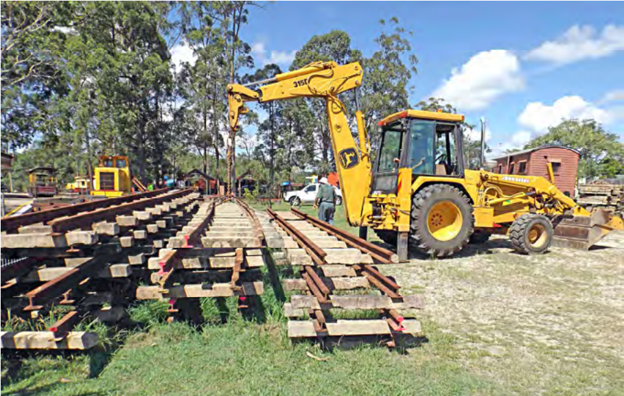
Ralph Cumner's backhoe sorting and selecting panels of track at Margaret Street, 5 April 2014. Greg Stephenson photographer.
