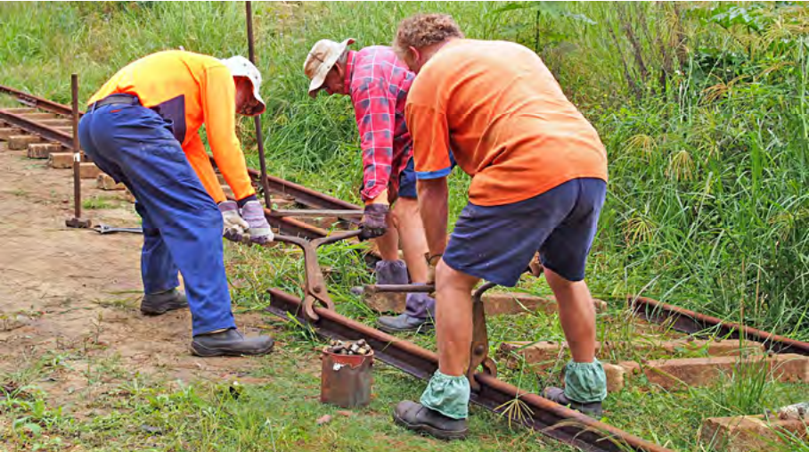
Kerry Rasmussen, Steve Baker and Dave Carusso positioning a rail before lifting it onto the sleepers, 14 June 2014. Sue Rasmussen photographer.
