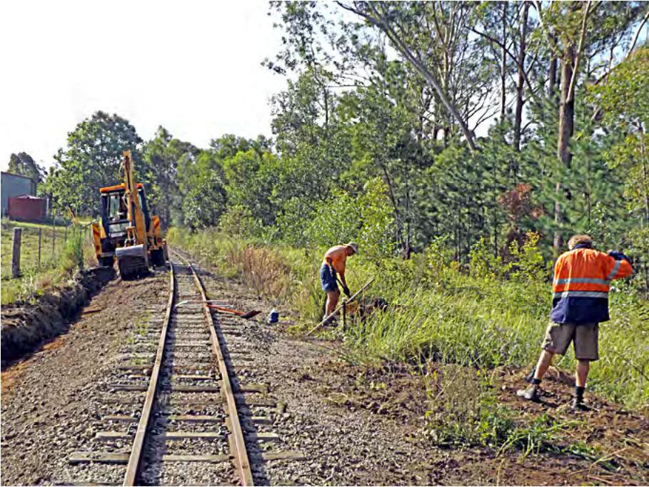
Ralph Cumner excavating the drain at Ch 550 whilst Steve Baker and Dave Caruzzo level out the excavated spoil. Greg Stephenson photographer.
