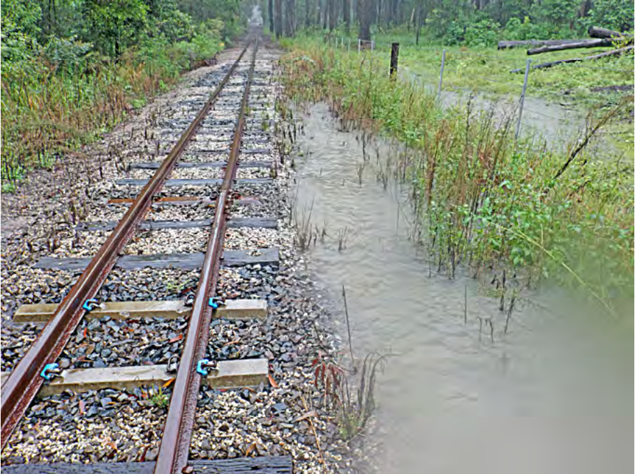
Water approaching rail level near Ch 550 on 21 February 2015 following cyclone Marcia. Greg Stephenson photographer.
