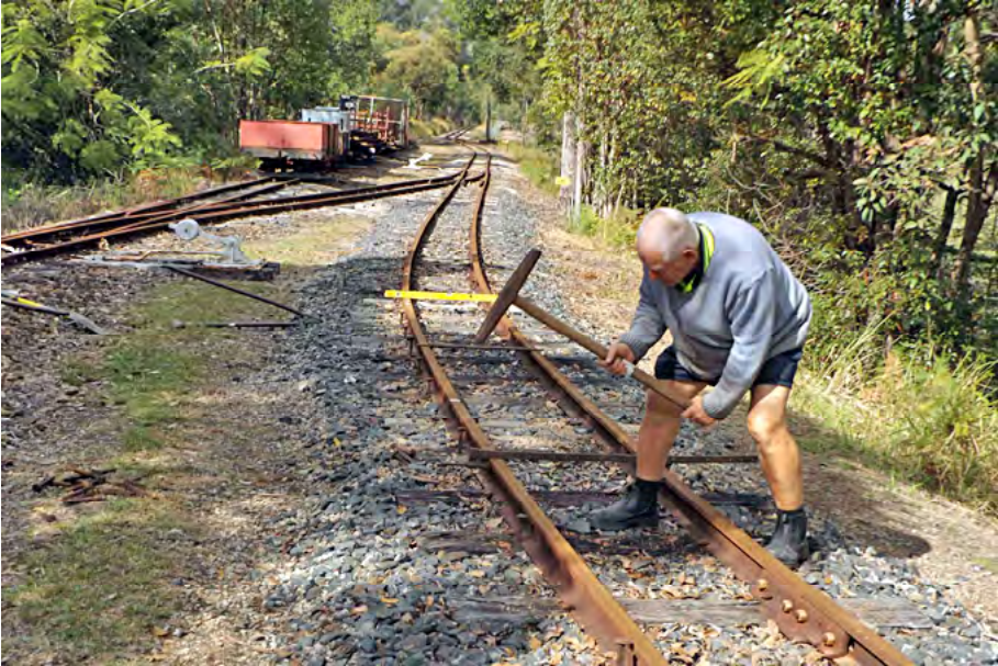
Re-spiking timber sleepers for mainline maintenance: Dave Pearson with spiking hammer, 27 June 2015. Greg Stephenson photographer.
