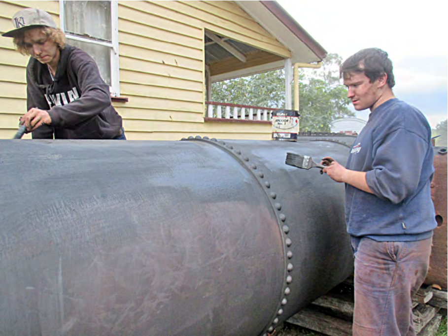
Aaron and Curtis painting the boiler with the boiler paint. Ryan Silk photographer.
