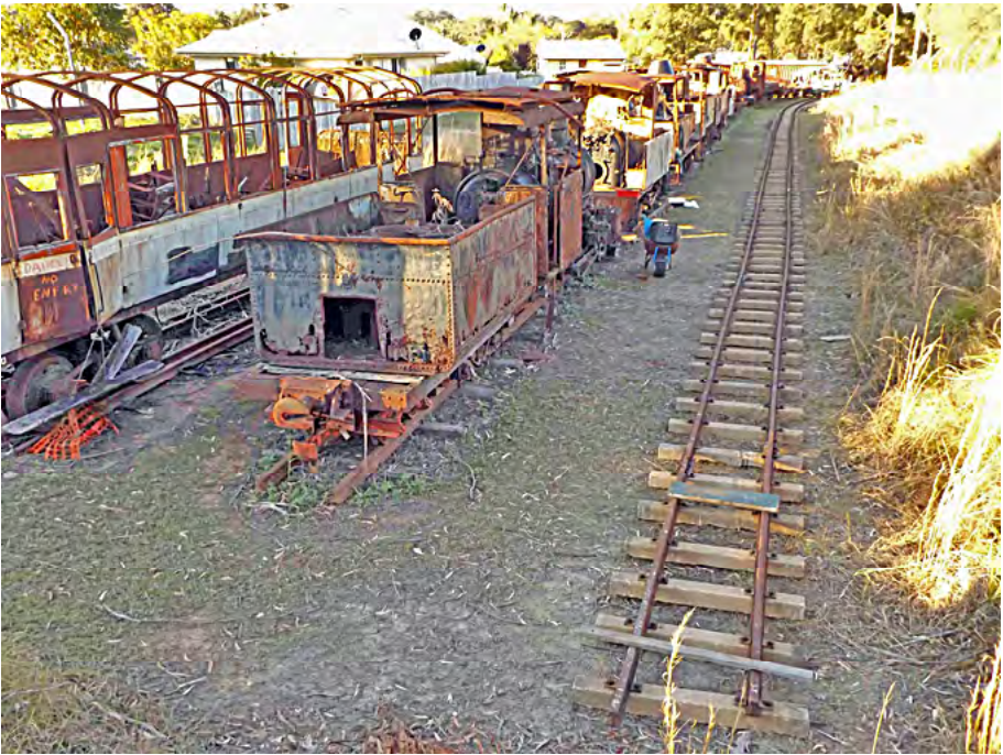
Another view of the completed storage siding ready for placing of rolling stock from the area of the new shed. Greg Stephenson photographer.
