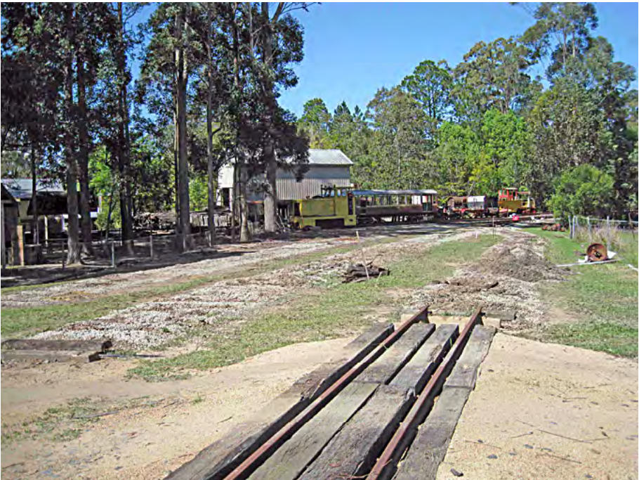
New shed site after removal of the existing track. Terry Olsson photographer.
