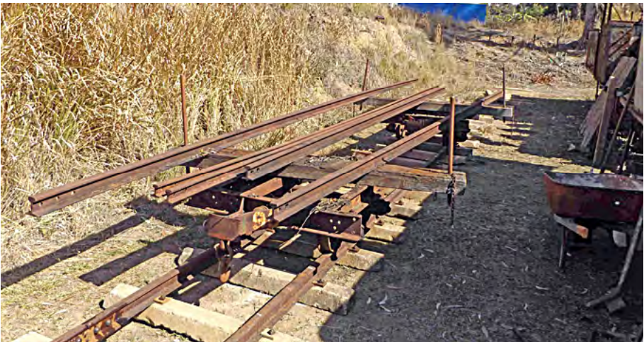
Bolster wagon of rails ready to be placed onto the concrete sleepers. Greg Stephenson photographer.
