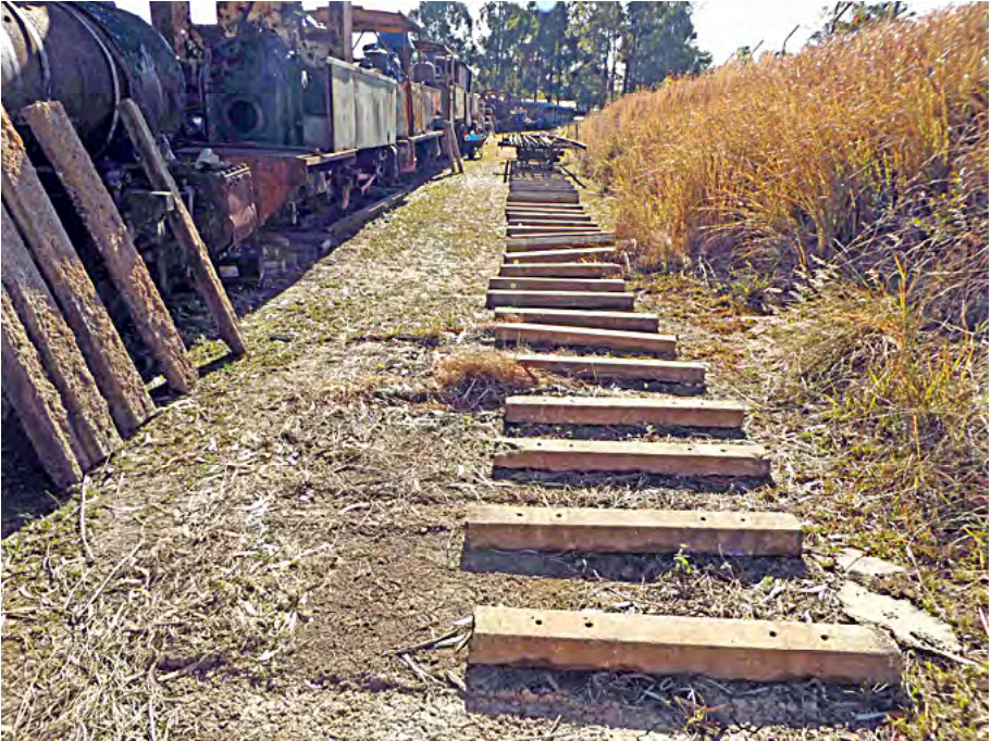
Concrete sleepers in place with bolster wagon of rails ready to be placed onto the sleepers. Greg Stephenson photographer.
