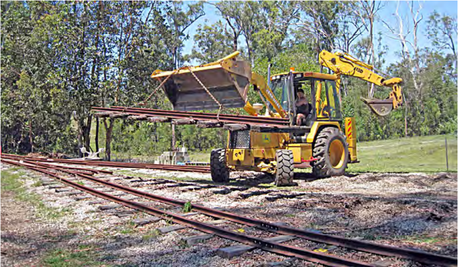
Ralph Cumner using his back hoe to remove panels of track in preparation for earthworks for the storage shed, 3 October 2015. Terry Olsson photographer
