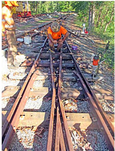
Photo right: Replacing point timbers with steel sleepers on points leading to the new storage shed. Greg Stephenson checks the gauge of the points as Harrison Silk watches. Magnetic base drill is sitting on timber sleeper in foreground. Ryan Thomas photographer.
