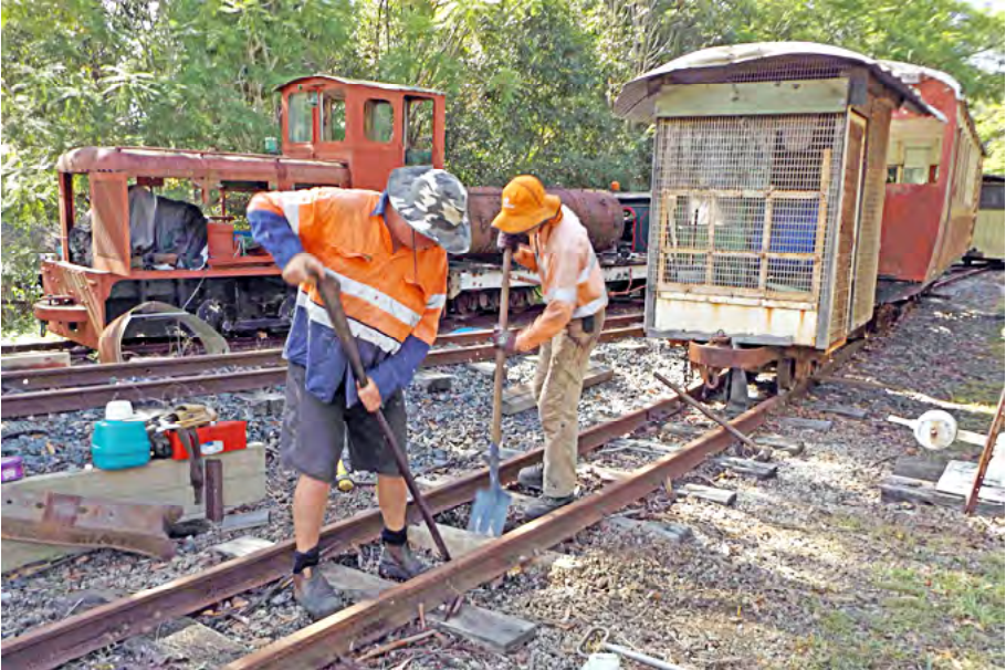
Dave Caruzzo and Harrison Silk insert a concrete sleeper into a workshop siding on 16 April 2016. Greg Stephenson photographer.
