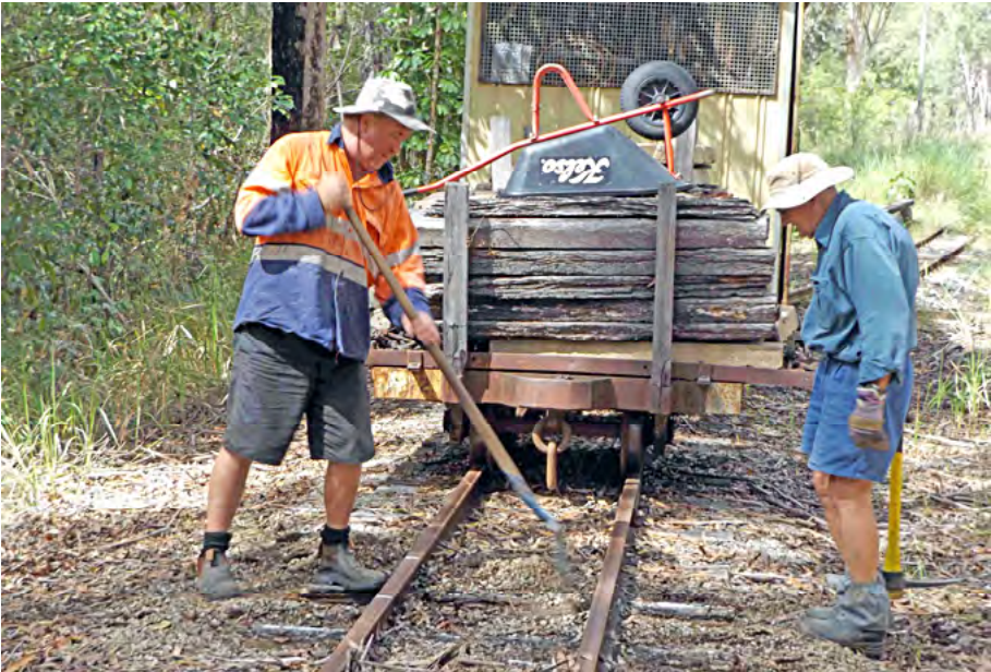
Dave Caruzzo and Steve Baker removing rotten timber sleepers at Ch 750 to allow replacement with concrete sleepers on 16 April 2016. Greg Stephenson photographer
