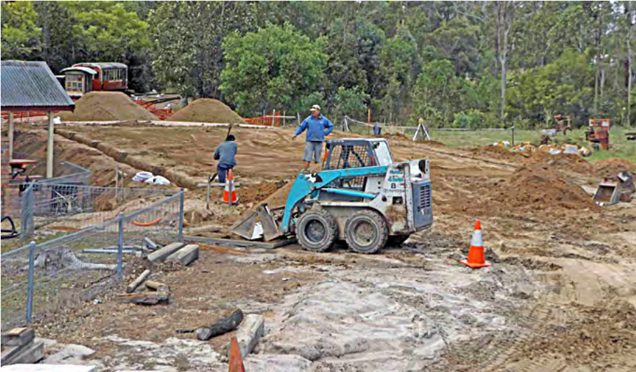
View on Wednesday 22 June 2016 from the verandah of the QCWA cottage of the foundation excavation for the locomotive storage shed being undertaken. Greg Stephenson photographer.
