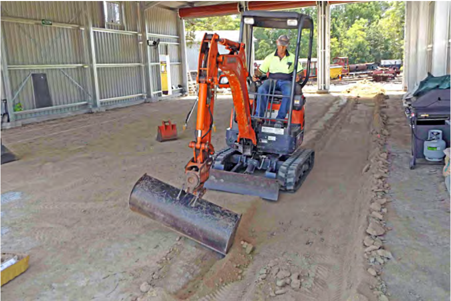
"Dingo Pete" using his mini-excavator to trim the batters of the excavation for the first rail line in the locomotive storage shed on 14 January 2017. Greg Stephenson photographer.
