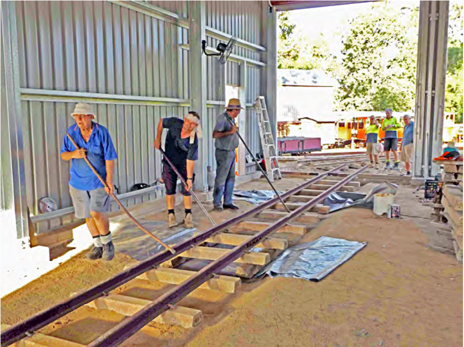
Bob Gough, Wayne Harmen and Morrie Mason using crow bars to adjust the alignment of the track panels prior to concreting the floor of the locomotive storage shed. Greg Stephenson photographer.
