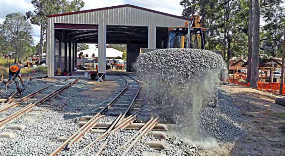
Ralph Cumner using his backhoe to transport and place ballast on Number 3 road. To reach this location, he travelled through the shed and along the track, 10 June 2017. Greg Stephenson photographer.
