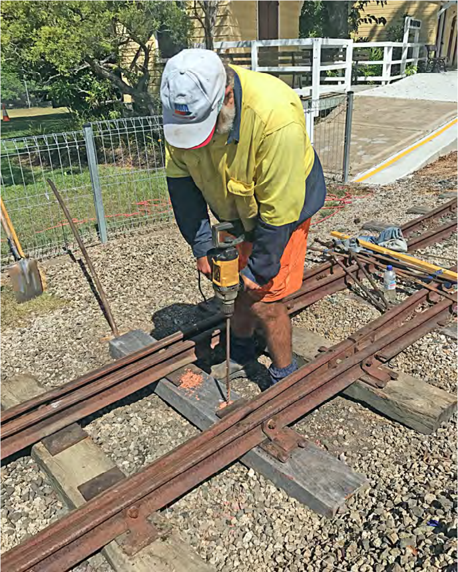
Greg Stephenson drilling the timber replacement sleepers at the Margaret Street passing loop points, 26 January 2019. And don't forget, we used to drill all these holes with a hand drill! Terry Olsson photographer.
