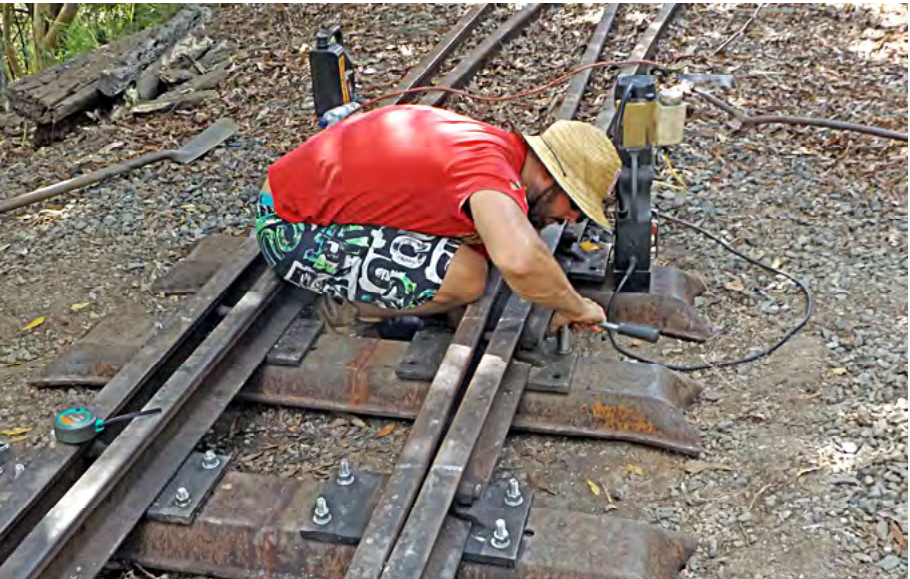
Samuel Erb using the magnetic base drill on the new steel sleepers (TOP) and bolting the chair plates to the new steel sleepers (BOTTOM) on the Mainline to Workshop points, 9 February 2019. Greg Stephenson photographer.
