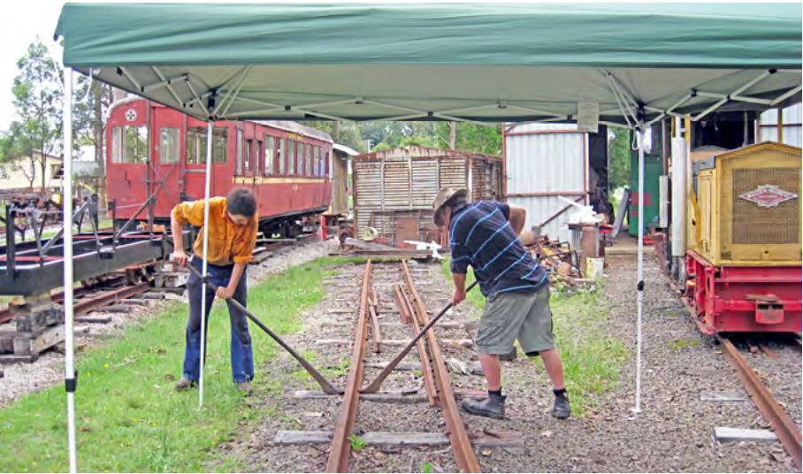
Dave and Ryan dismantling the workshop area's storage siding in preparation for the new service track, 12 December 2010. Terry Olsson photo.
