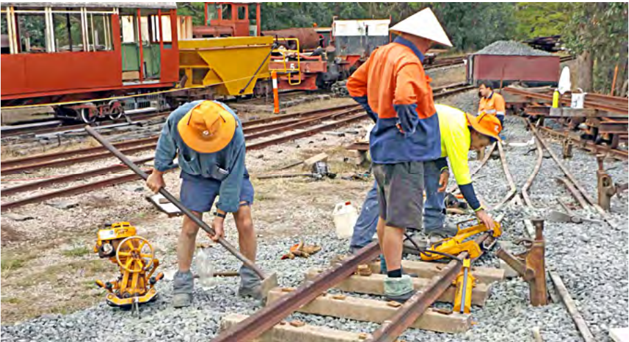
Steve Baker uses a bar to adjust the position of ex-Ingham concrete sleepers on Number 3 road, whilst Dave Caruzzo and Terry Olsson use the hydraulic rail bender to adjust the alignment of the rails at the joint, 17 June 2017. In the background, Ryan Thomas is fitting rods to the point levers. Greg Stephenson photographer.
