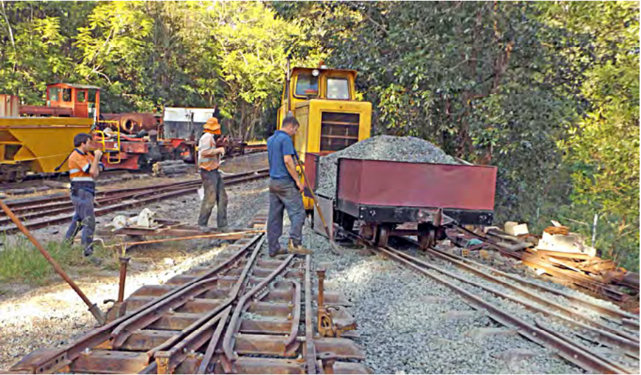
"Gemco" was used to bring a load of ballast in the ex-Douglas Shire Tramway wagon along Number 1 road so that points between Number 2 and 3 roads can be ballasted. The pointwork has been lifted to the correct height and supported on jacks, 3 June 2017. Greg Stephenson photographer.
