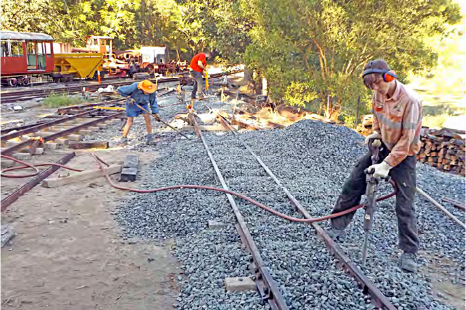
Harrison Silk, Steve Baker and Tyler Meiklejohn packing ballast on Number 1 road to new locomotive storage shed, 27 May 2017. Greg Stephenson photographer.
