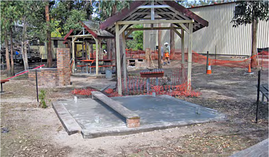
Concreting the base for the relocated picnic shelter, 30 September 2017. Terry Olsson photographer.
