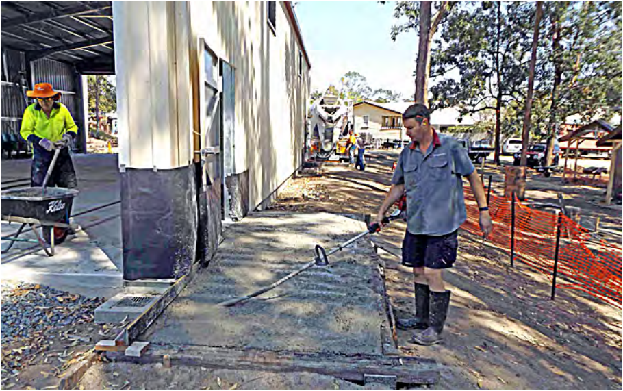
Wayne Harman vibrating concrete on the access ramp nearest the main line whilst concrete is placed in the other access ramp, 30 September 2017. Greg Stephenson photographer.
