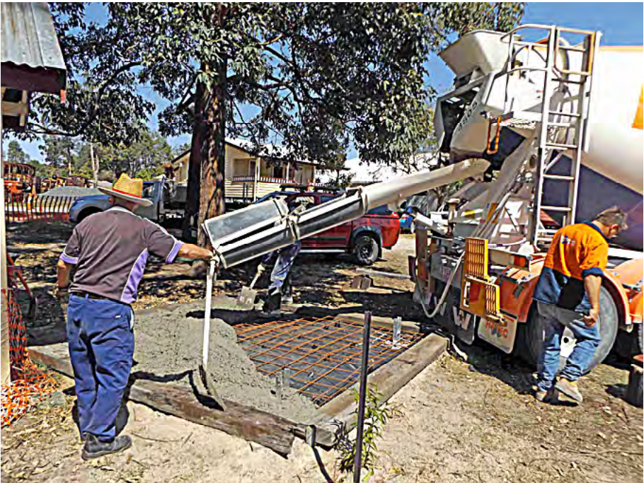
Placing concrete in the slab for the relocated picnic shelter, 30 September 2017. Greg Stephenson photographer.
