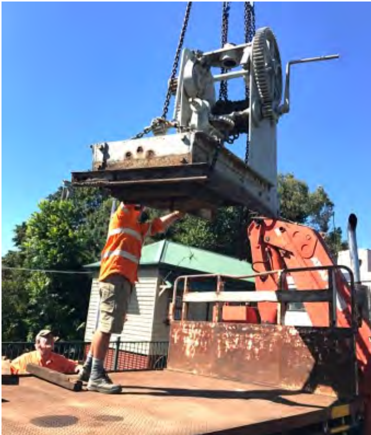
Getting the Cooroy goods crane donated by Nambour Historical Society loaded for transport to Woodford, 5 April 2023. Terry Olsson photographer.
