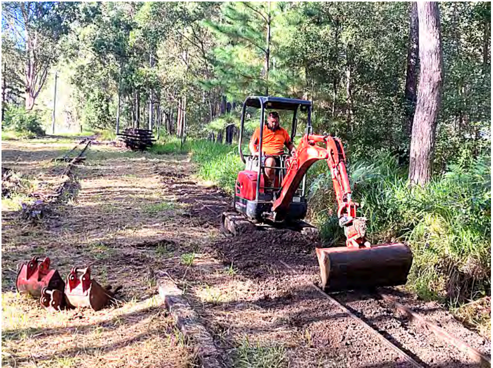
Tim from Cosmos Earthmoving clearing old ballast from the future passing loop at Peterson Road Station, 11 May 2024. Greg Stephenson photographer
