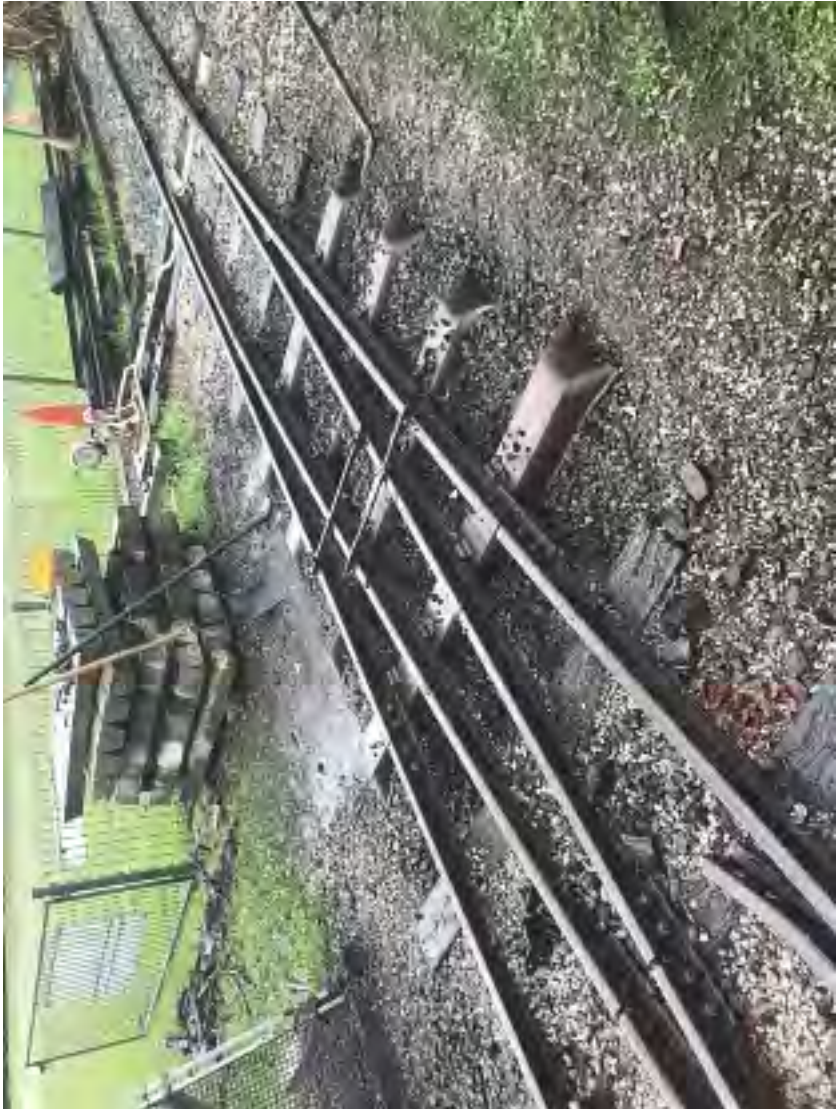
Trackwork Saturday: the points to the Woodford station headshunt, 12 April 2025. This set of points contains the last timber sleepers in the mainline, the rest of it is now all concrete or steel sleepers. Terry Olsson photographer.
