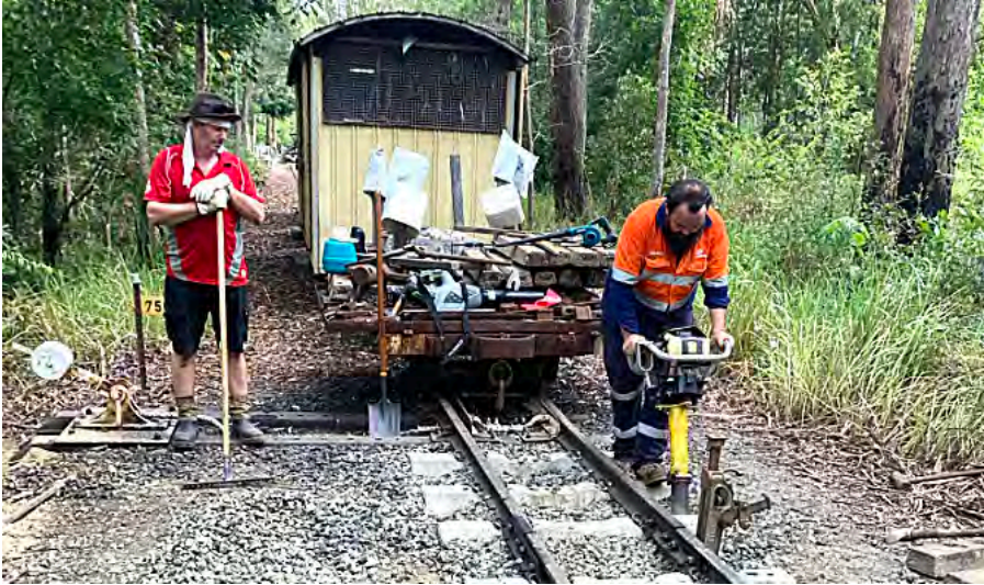
Ryan Thomas packing ballast whilst Wayne Harman replaces the ballast removed as part of the regauging the joint at the start of COVID Junction, 10 January 2026. Greg Stephenson photographer.
